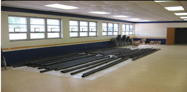
A small sample of the pipe used in the sprinkler system is laid out in room 121.
